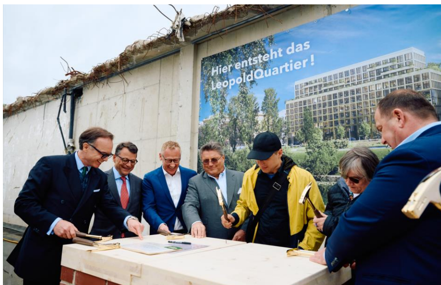
Laying of the foundation stone at Vienna's urban development area LeopoldQuartier © Philipp Horak
