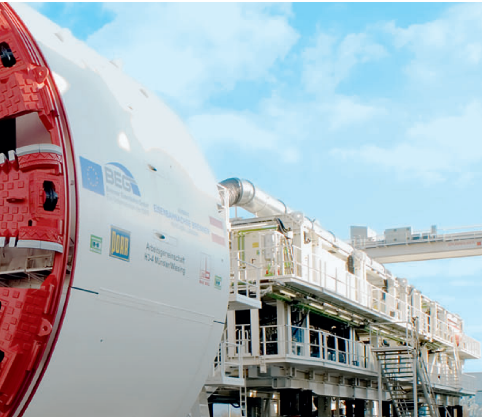
Slurry shield tunnelling machine used on the Münster-Wiesing project unit in the Tyrol, 2007
