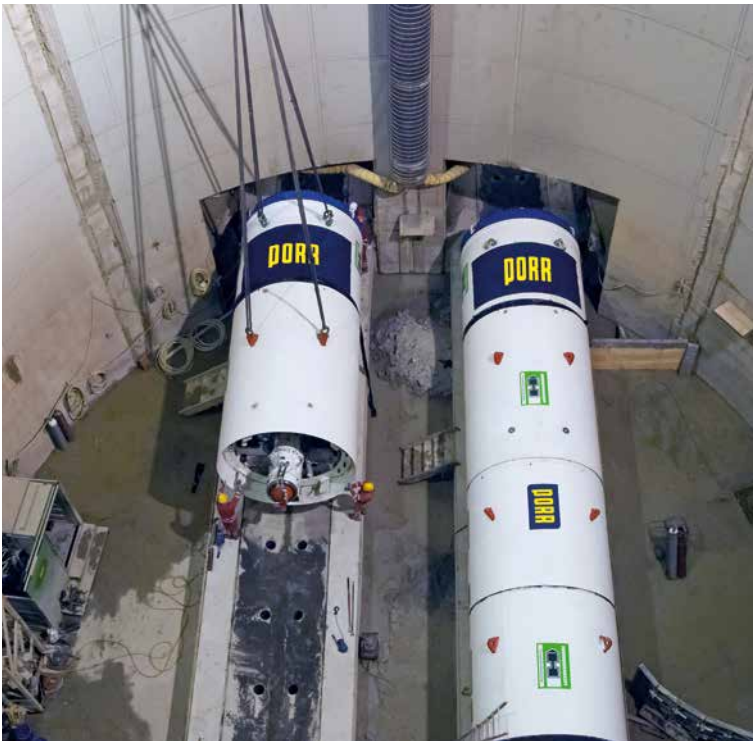
Emscher Section 40 Assembling the second EPB shield machine to build the 10km long waste water duct through the Ruhr area
