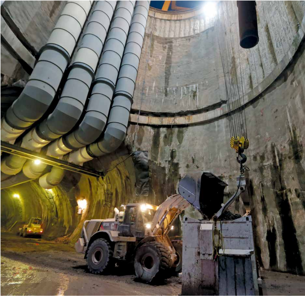
Stuttgart 21 . Obertürkheim and Untertürkheim construction sections The Ulmerstrasse shaft was used for supply and spoil removal for four advances
