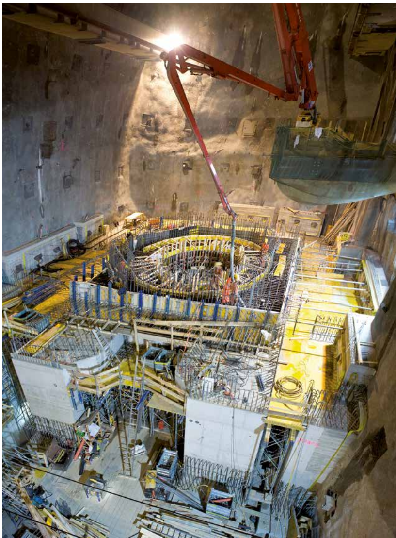
Limberg II pumped-storage power plant A 62m long, 25m wide and 43m high cavern was excavated inside the mountain for the two 240MV machines
