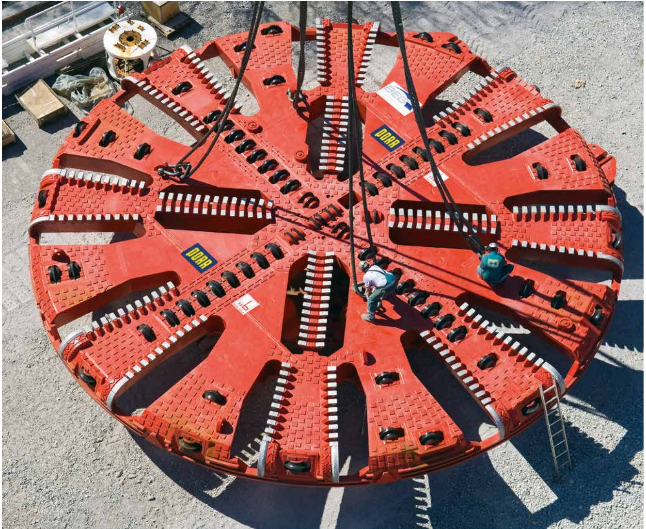
Lower Inn Valley Railway . Section H3-4 Precision work assembling the 230t cutter head on the tunnel boring machine
